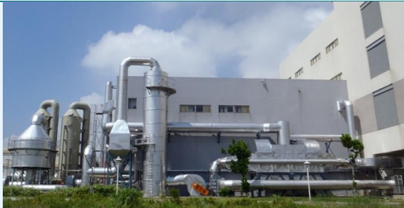
VOC Condensation & Concentration System
